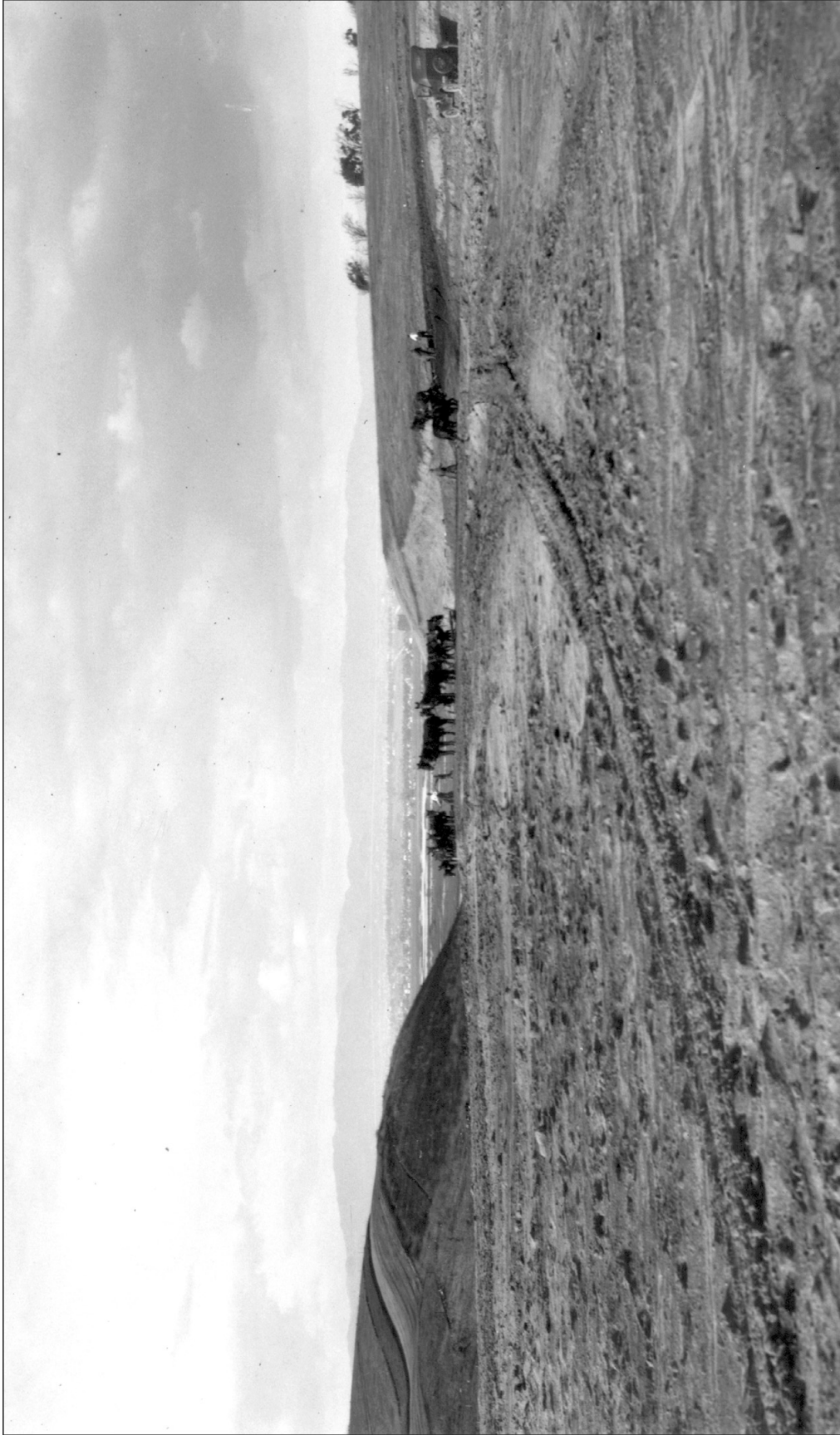
Figure 15. 1927 view to the north during grading for Lincoln Boulevard above the Lincoln Gap (courtesy of the Automobile Club of Southern California Archives).
